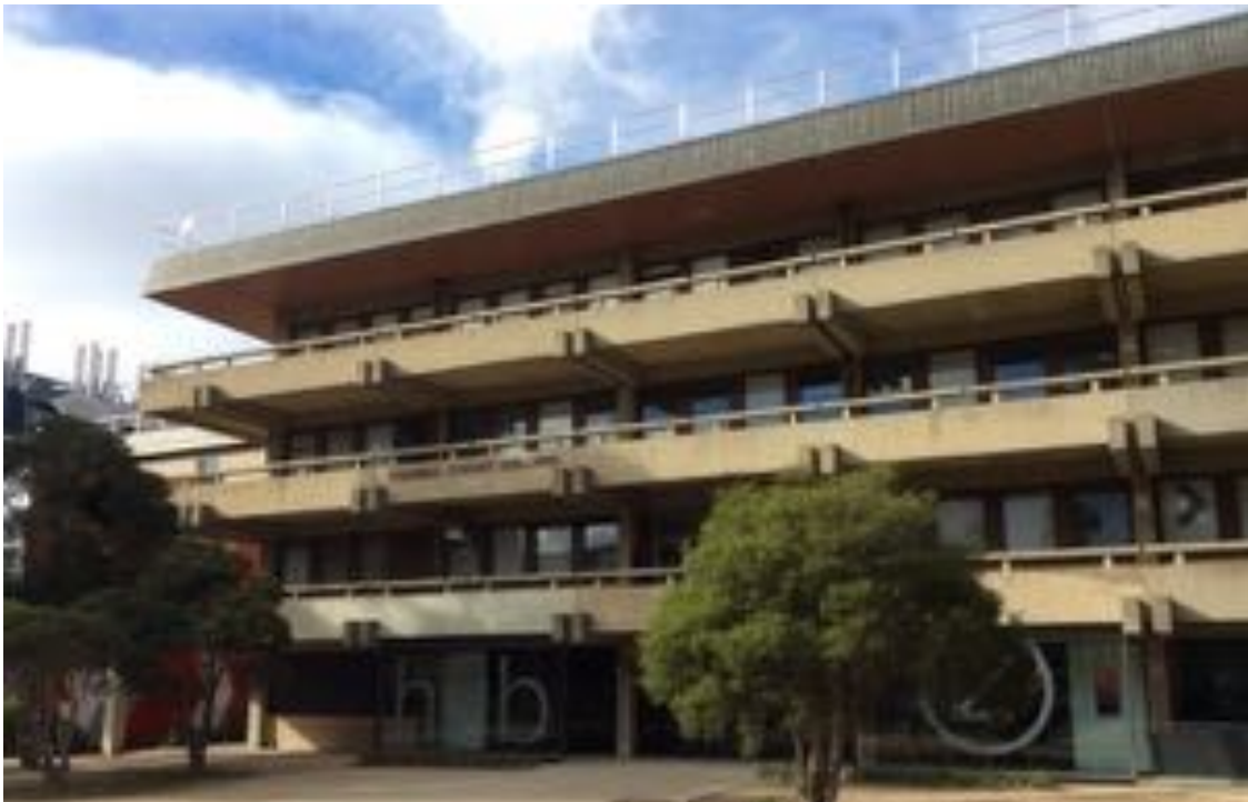
The Thomas Cherry Building – the home of the School of Agriculture for its early years.
